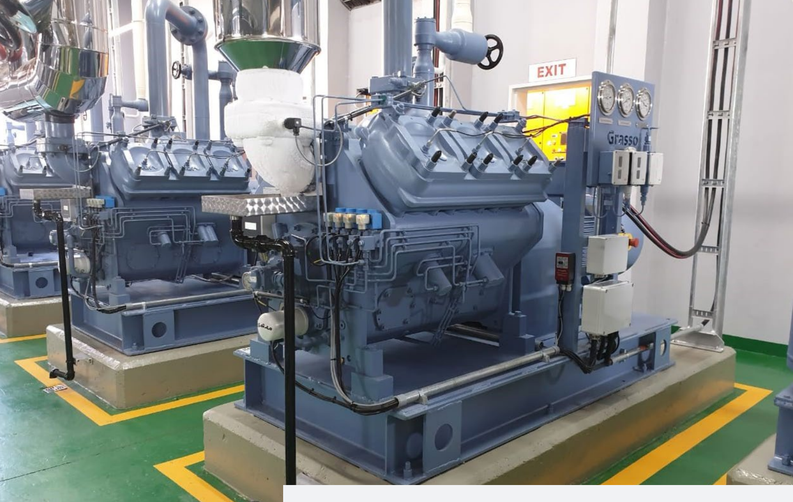
The ammonia compressors up close
